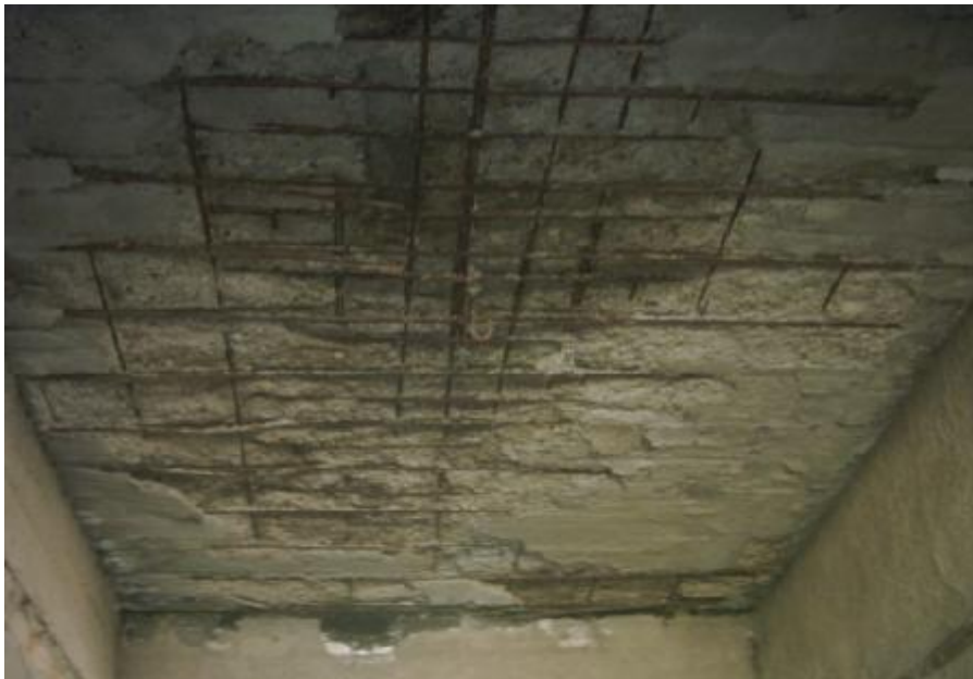
Figure 4 show the severe damage in slabs [Anbar Rehabilitation unite]
