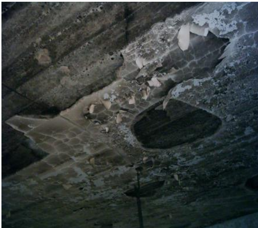
Figure 5 show the Simple damage in slabs [Anbar Rehabilitation unite]
