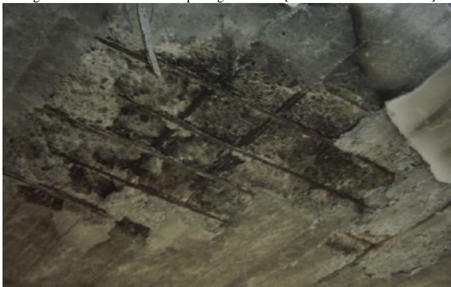
Figure 3 show the moderate damage in slabs [Anbar Rehabilitation unite]
