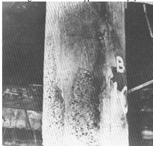
Figure 2 show the cracks and spalling in column [Anbar Rehabilitation unite]
